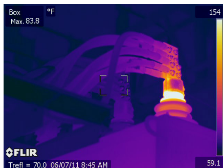
Overheated Transformer Bushing
